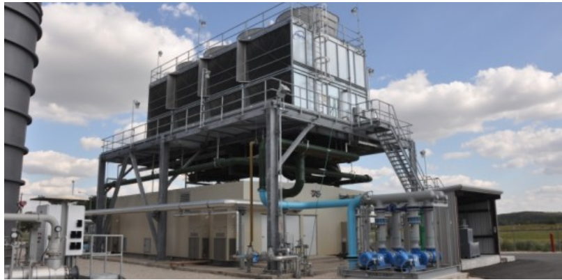
Figure 2-9: Typical turbine air chilling system with water cooling tower mounted above the chiller & pump house (Turbine Air Systems)
